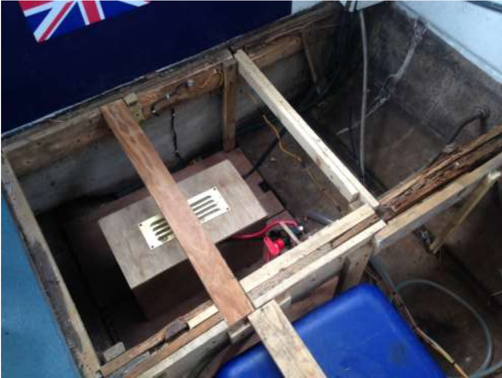
Beneath the cockpit decking mixture of rotten wood and pallet wood.
