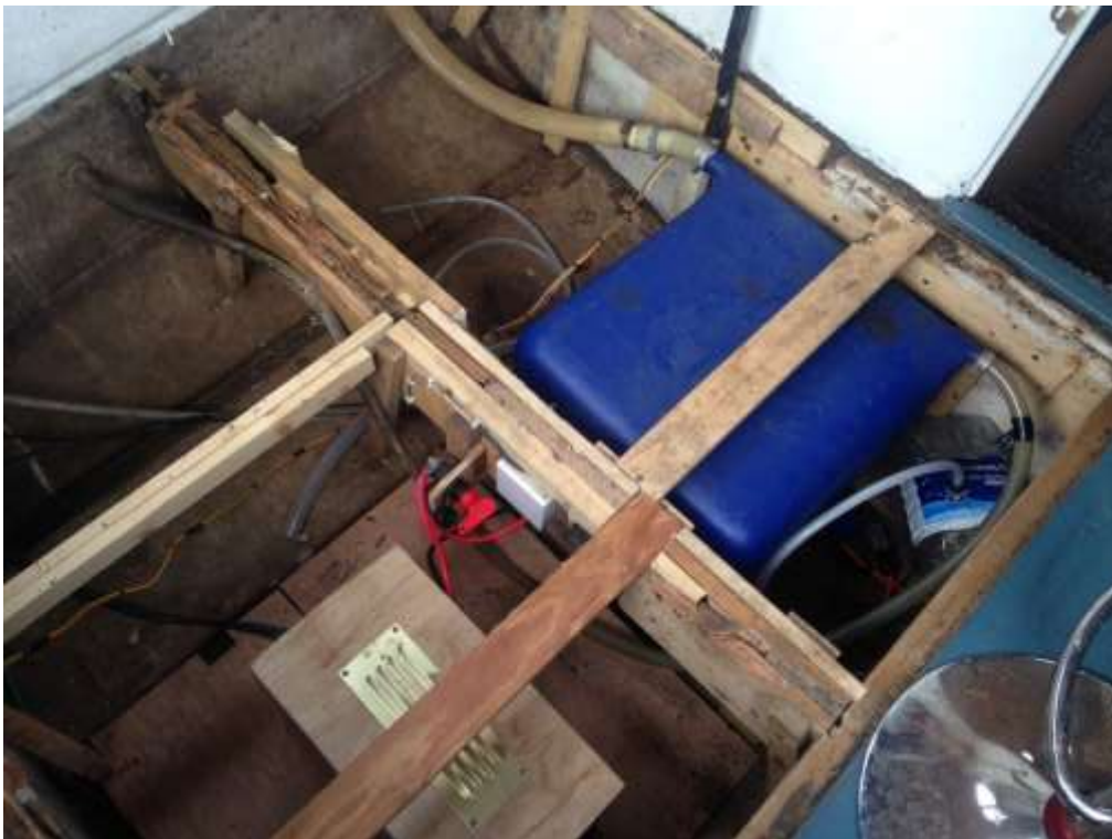
Fresh water pump removed as a missing fitting was leaking. Will order and fit new pump.
